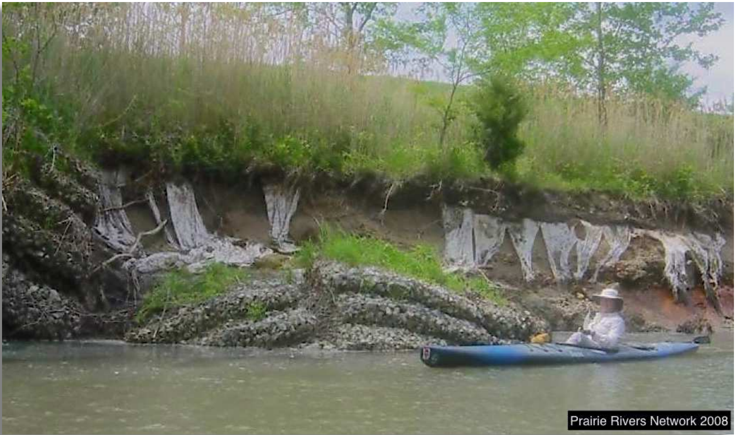
The river is eroding the walls of these pits. Gabions installed to shore up the banks are failing.
