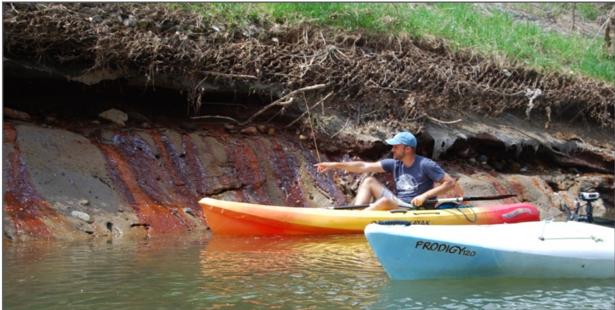
Coal ash pollution seeping out of banks of the Middle Fork of the Vermilion River is visible in areas where gabions, installed to stop erosion, have failed. Photo by EJC.
